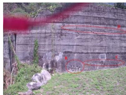
Figure 8: Visible light image at dam wing in area B~D
